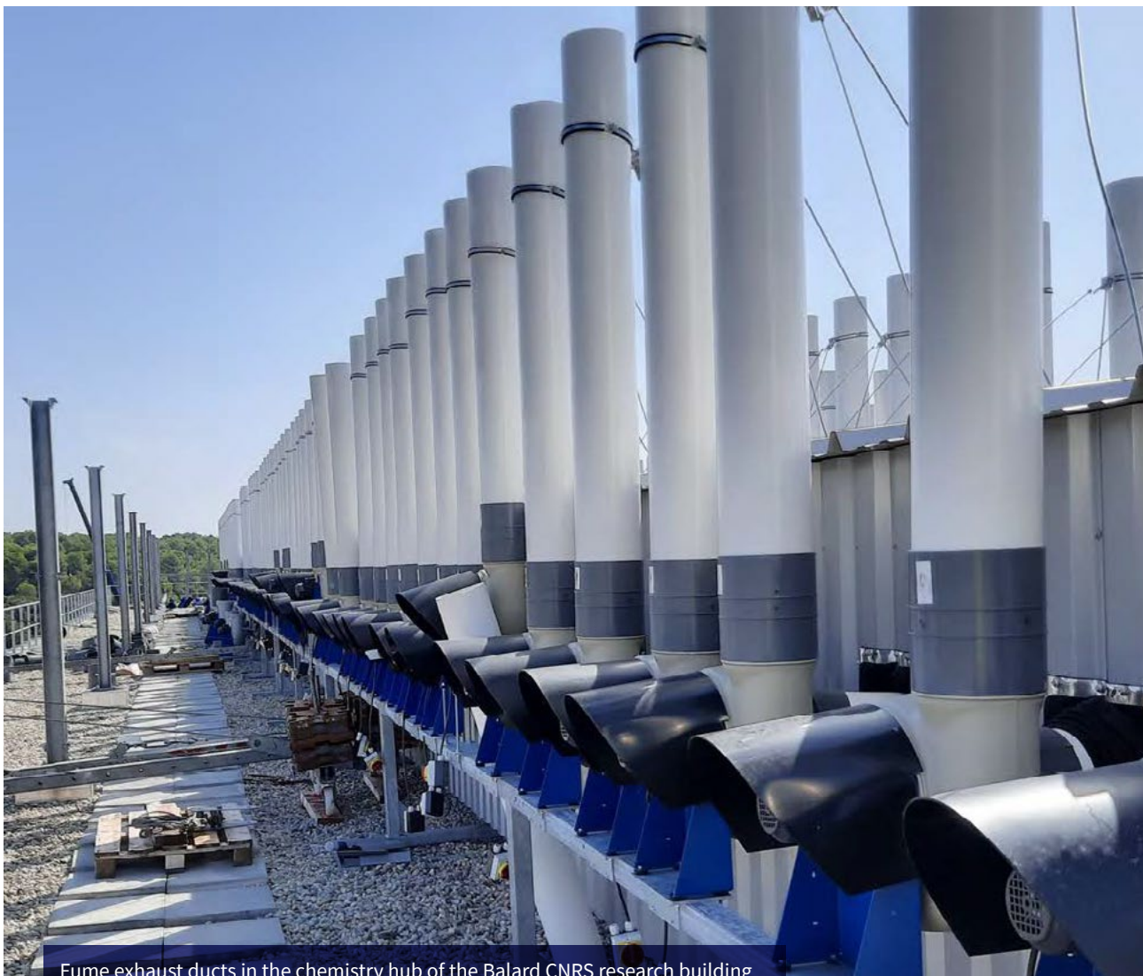
Fume exhaust ducts in the chemistry hub of the Balard CNRS research building
