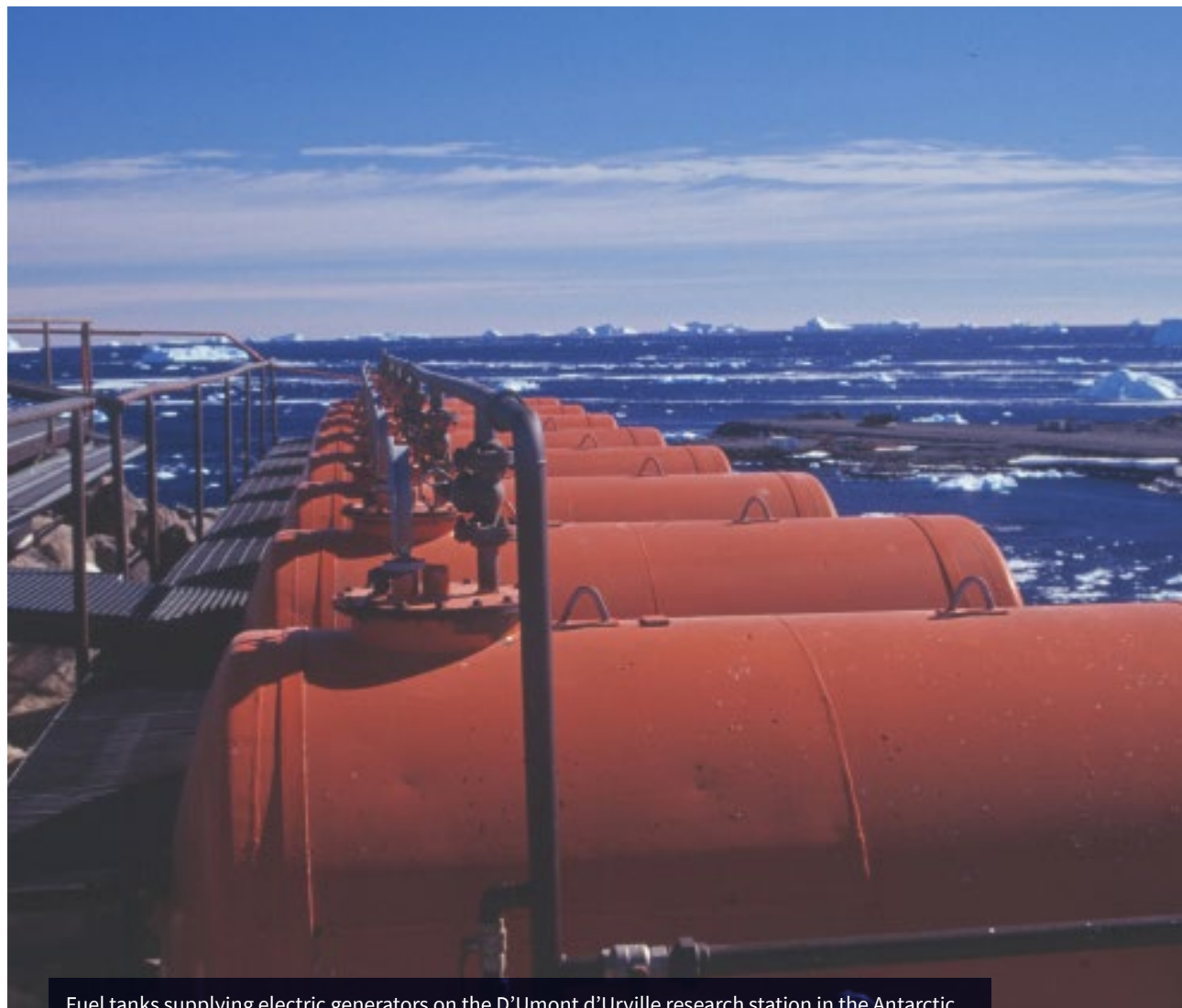
Fuel tanks supplying electric generators on the D'Umont d'Urville research station in the Antarctic
